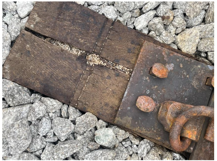
Pellets observed within aggregate bordering track
